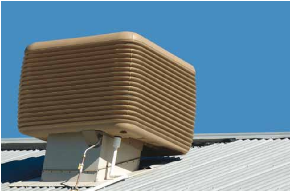
The main unit of an evaporative air-conditioner is usually located on the roof
