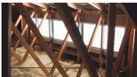
This example shows bulk ceiling insulation and reflective foil on the inside of the roof
