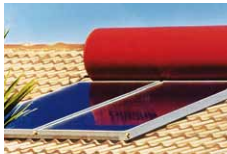
A solar hot water system will generally have solar collector panels on the roof
