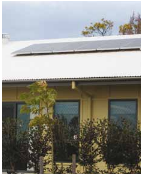
Solar power systems can be identified by a collection of solar panels on the roof
