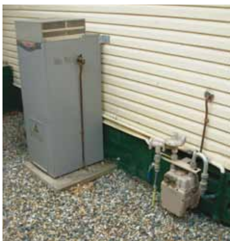
An example of a storage gas hot water system
