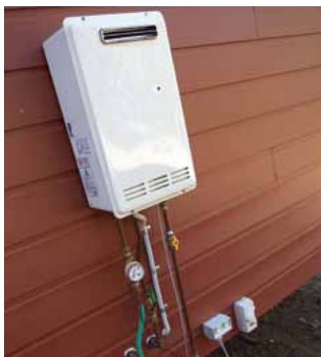
An instantaneous gas hot water system
